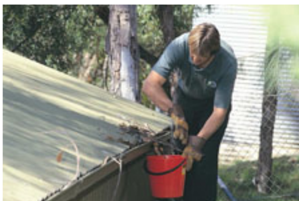
Clean gutters of leaves and other debris
